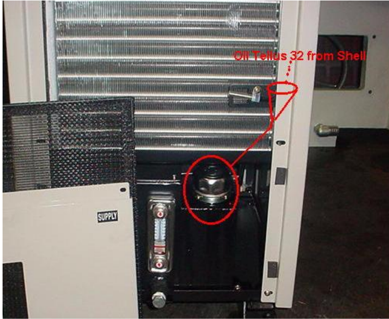
Oil spindle chiller Kaukan-4pts on the floor
